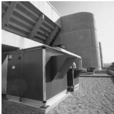
Air conditioning application
